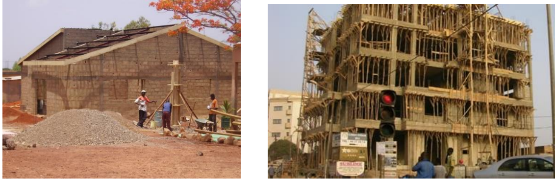
Figure 15 In many countries, CHB is widely used both for small buildings (left) and middle/high rise buildings(right) in Burkina-Faso. There are problems in quality especially blocks manufactured by contractors in construction site (not by manufactures in manufacturing plants) and skills of workers. (Report on the project “Safer CHB Construction in the Philippines”, March,2023, Hokkaido Building Engineering Association (HoBEA) 7.3.4 Problems on CHB spreading in wider regions in the world)
