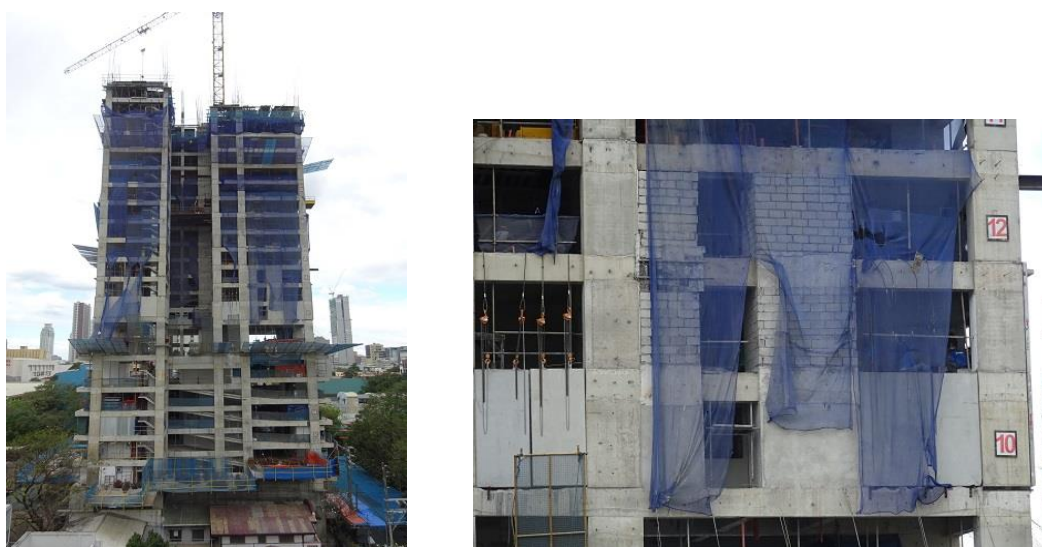
Figure 2 High-rise building under construction in Metro Manila. Left: view of the total structure, Right: detail of the buildings. CHB is used for outer walls.
