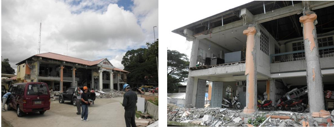
Figure 6 Heavily damaged building by the Bohol earthquake 2013. Left: view of total building of municipal government office of Sagbayan, the Philippines, Right: Close-up view of the building in the left. Outer non-structural CHB walls were completely destroyed.
