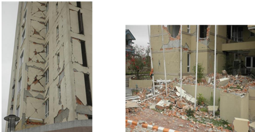
Figure 16 Damage in non-structural walls by Gorkha Earthquake 2015. Most of non-structural walls (non-reinforced brick walls) in modern high-rise apartments were damaged. Left: shear cracks in non-structural walls, Right: debris of non-structural wall falling down to the ground
