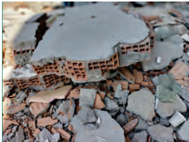
Damaged nonstructural infill brick wall (2023 Turkey Earthquake)
