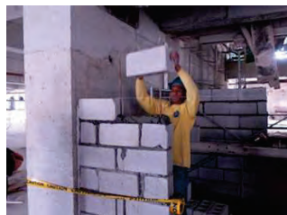
Conventional way of block laying in the Philippines. Blocks must be raised up to the top of vertical rebar
